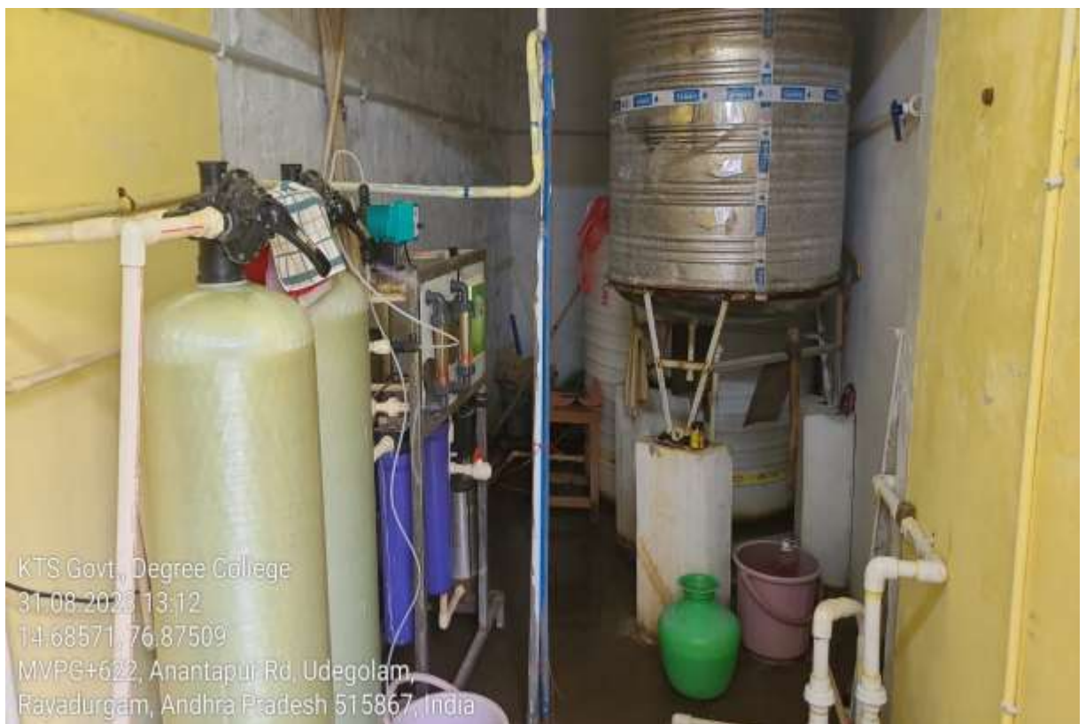
RO WATER PLANT
